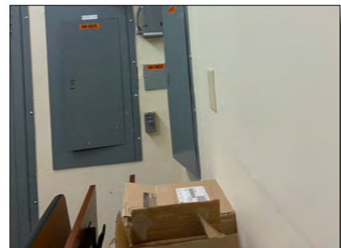
Relocate items stored in front of electrical panels
