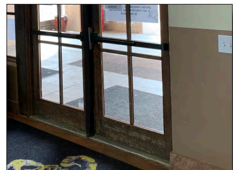
Repaint interior of main entry doors and install metal kick plates to protect from future damage
