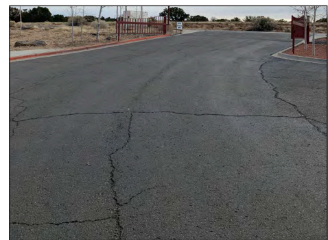
Southeast entrance to the site: multiple cracks in asphalt need repairs and seal coat
