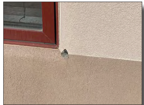
Damaged stucco along southside of building near Classroom #115
