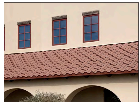
Exterior wood lintels and trim need to be repainted/ stained
