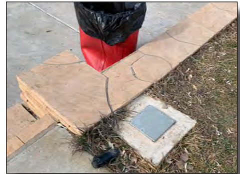
Broken sprinkler head: east side of building near play area
