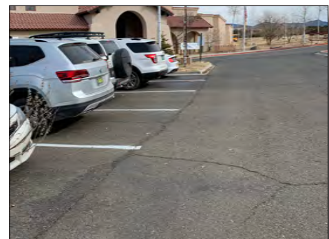
Parking lot areas also have a lot of asphalt cracks that need repairs and seal coat
